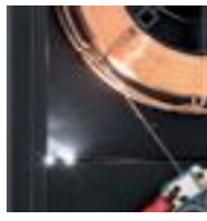
LED lighting inside feeder chamber
